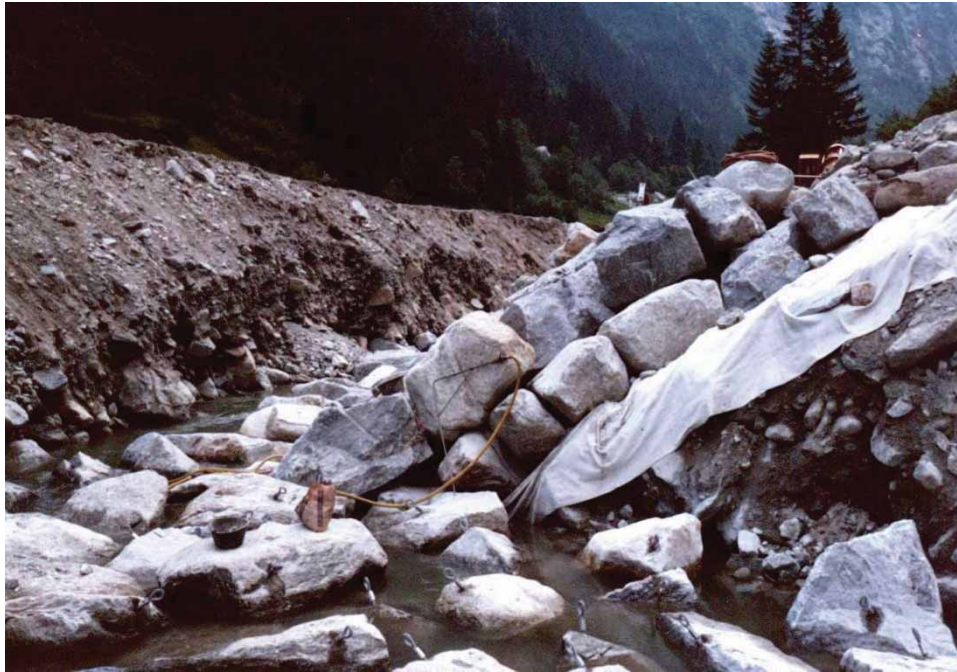
Figure 1 Riprap on the Reuss River in Switzerland under construction with individually placed large blocks in two layers on a geotextile. Block weight is 4.0–4.5 t. (Courtesy of A.J. Schleiss)
