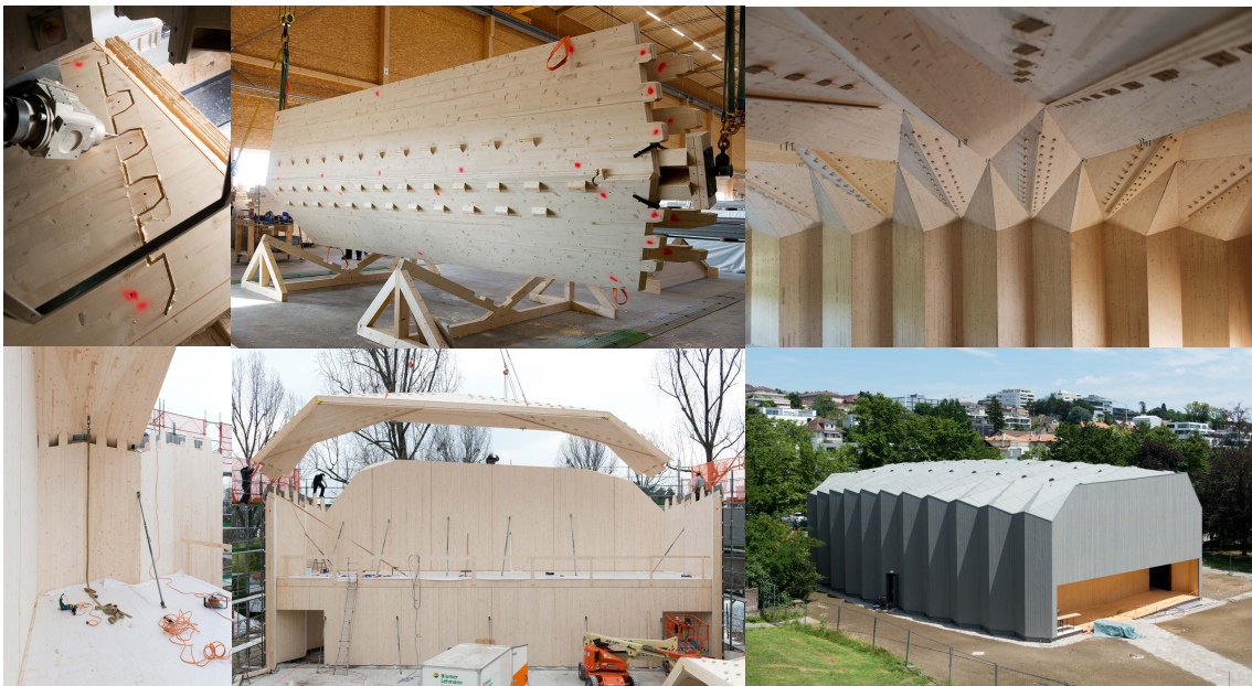
The new timber pavillon of the Vidy theatre (photo credit: Ilka Kramer)
